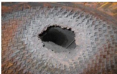
The fire burned a hole in the packing.
