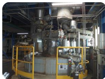
Batch reactor and handling raw materials
